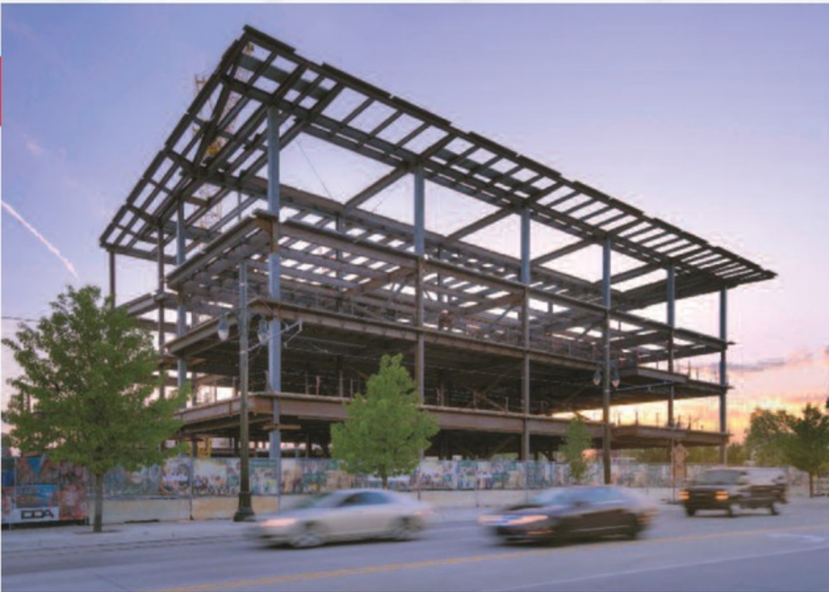
The Steel Challenge: Installing a complex, multi-dimensional, cantilevered canopy for this showcase, four-story building.
